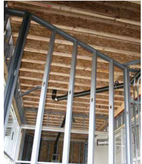
The project used light-gauge metal framing and plywood sheathing for the exterior walls.
