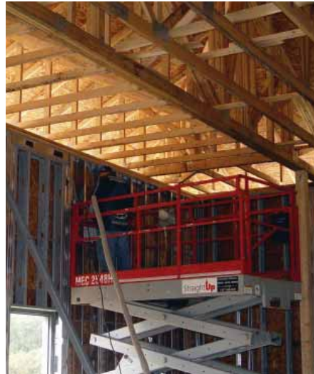
To achieve a low-profile roof line the design team incorporated wood I-joists and pre-engineered wood trusses.
