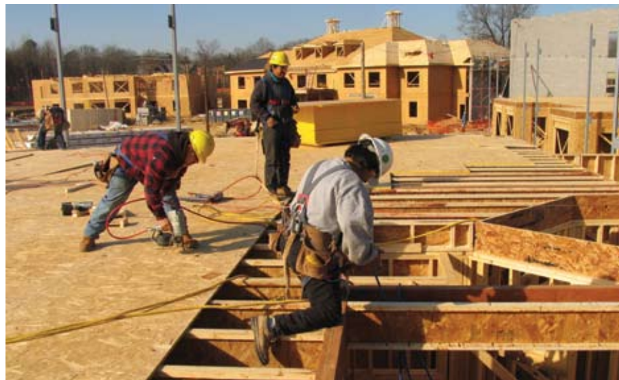
By using 11-7/8-inch-deep I-joists, the designers were able to address height restrictions in the floor-ceiling assemblies. I-joists also eliminated the need for sprinklers in the concealed spaces.
