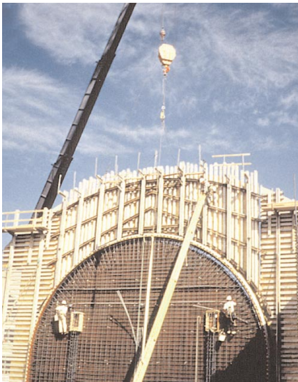
Over 4,000 sheets of HDO plywood were used to create sections of the giant gang forms.
